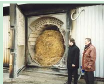
Straw combustion boiler in Juknaiciai boiler-house (thermal power of one boiler – 250 kW, four boilers installed, total power – 1000 kW)
