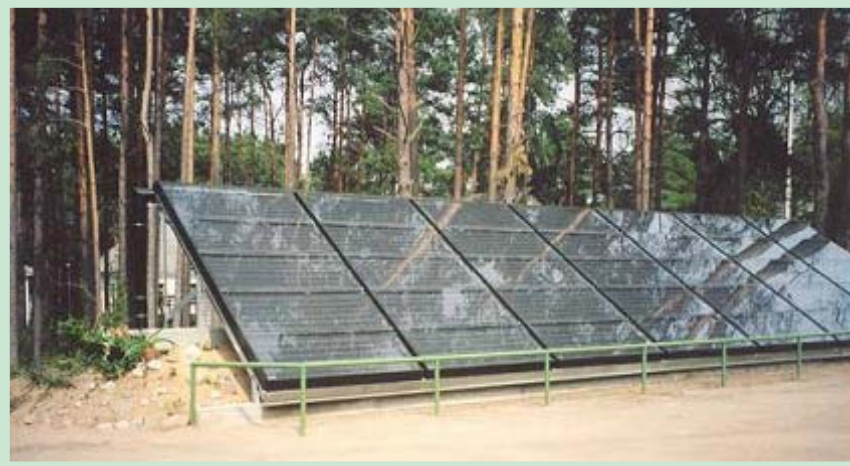
Solar collectors. SE Children's sanatorium of Kacergine
